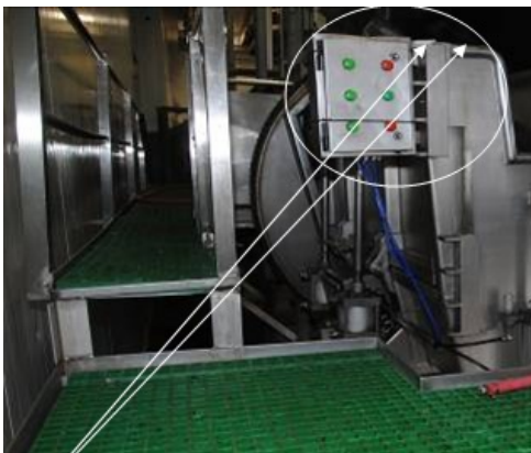
Area of the rotating knocking box where the employee became trapped
